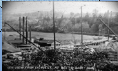
View from the West during dam construction. In the background are the Palisades.
