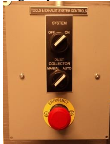
118B Emergency Power Kill Switch
