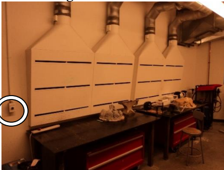
Welding Bench Slotted Hoods
